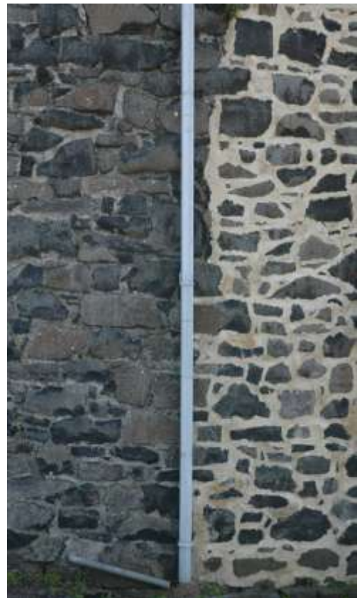
It is the stonework which should predominate (left) not the mortar (right)
