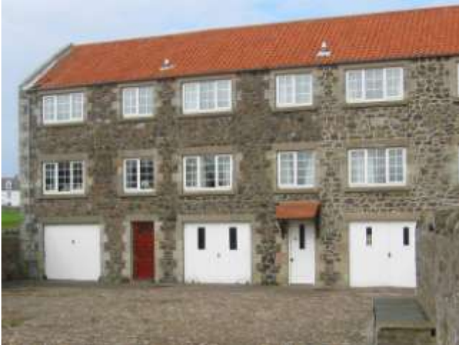
This three storey building can cope with the insertion of multiple garage doors
