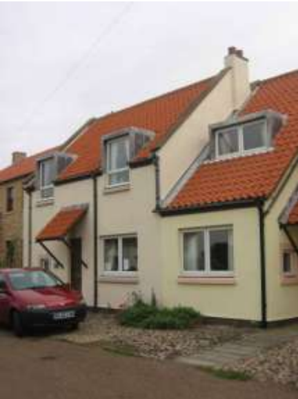
Square lead covered dormers – an alternative still subsidiary to the main roof surface
